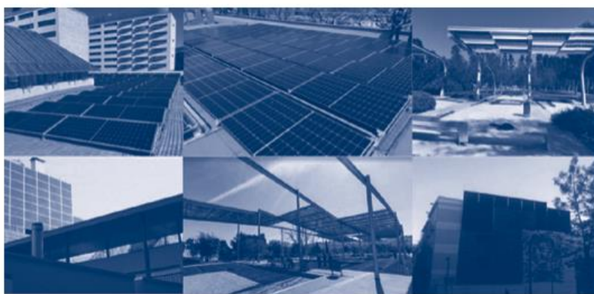
Image 1. Photovoltaic installations on municipal buildings
